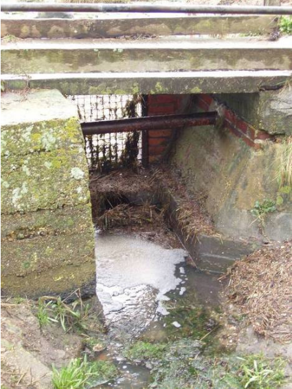
Shore Road Trippett pipe blocked 11 th March
