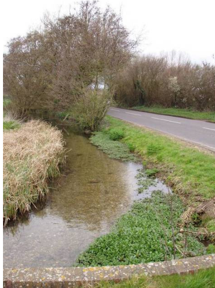
Ratham Lane – stream constricted by vegetation
