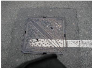
For ever flowing manhole at entrance to Crede Lane Bosham (off Walton Lane) Continual flow for over 12 months.
