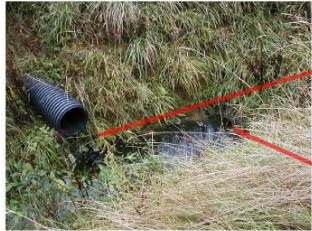
Overflow pipe from holding area flowing gently Entry pipe needs clearing
